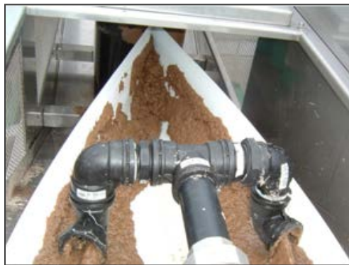
SLUDGE FEEDING INTO THE V-FOLD'S LEVEL CONTROLLED FEED CAVITY.
